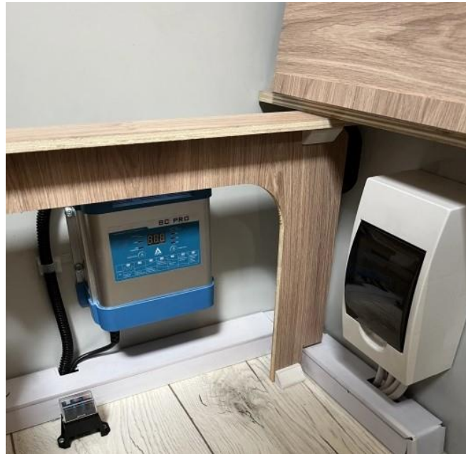
Figure 3-Power supply with switch cabinet
